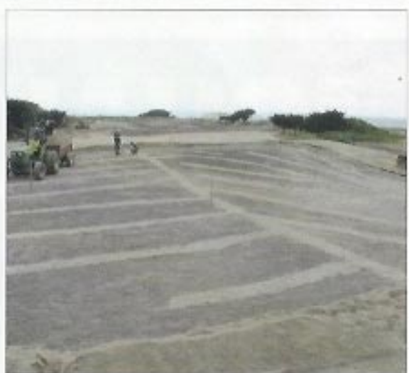
Pipe was laid every 12 feet under the fairways of the Shores Course to improve drainage.
